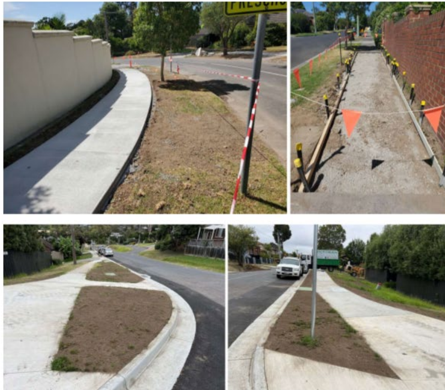
The footpath program is progressing very well with nearly all projects completed or on track and nearing completion including Wood Street pictured directly above.
