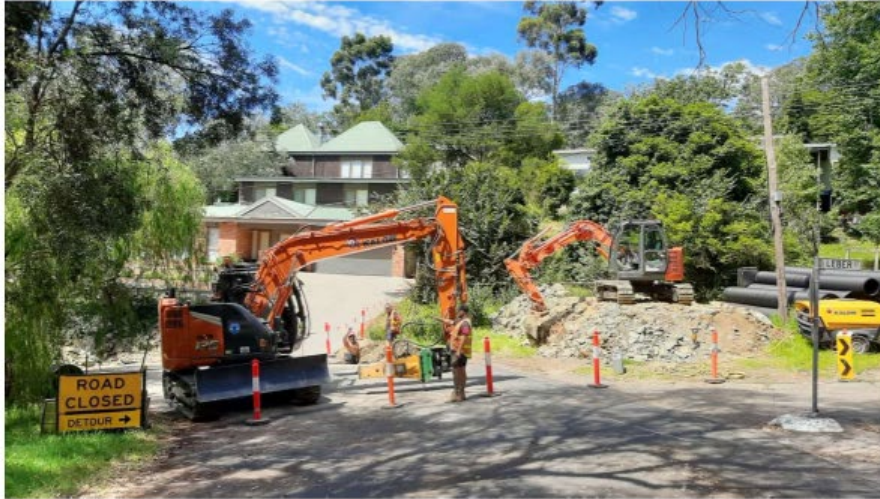
The overall drainage program is ahead of schedule for this time of year. Works at Melbourne Hill are shown above.
