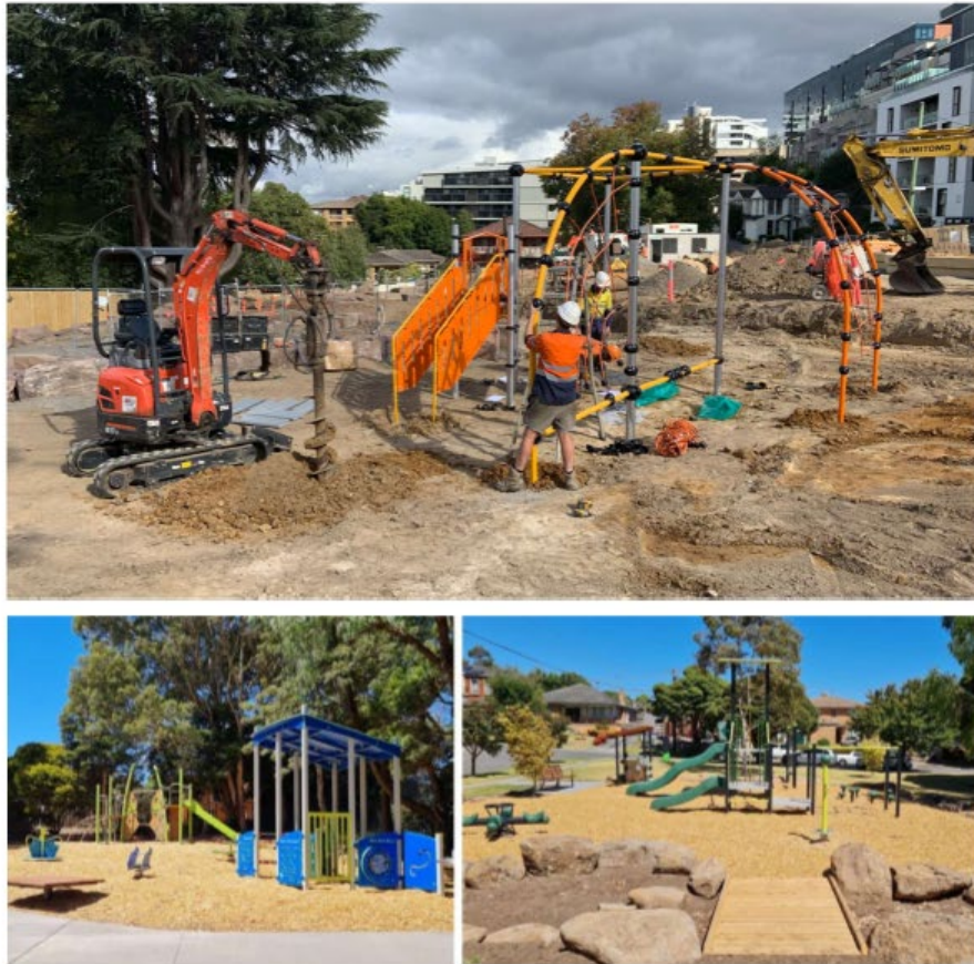
Work on the construction and renewal of play spaces is progressing well, with projects Hodgson and Swanson Reserve having reached completion and all other projects being on track.
