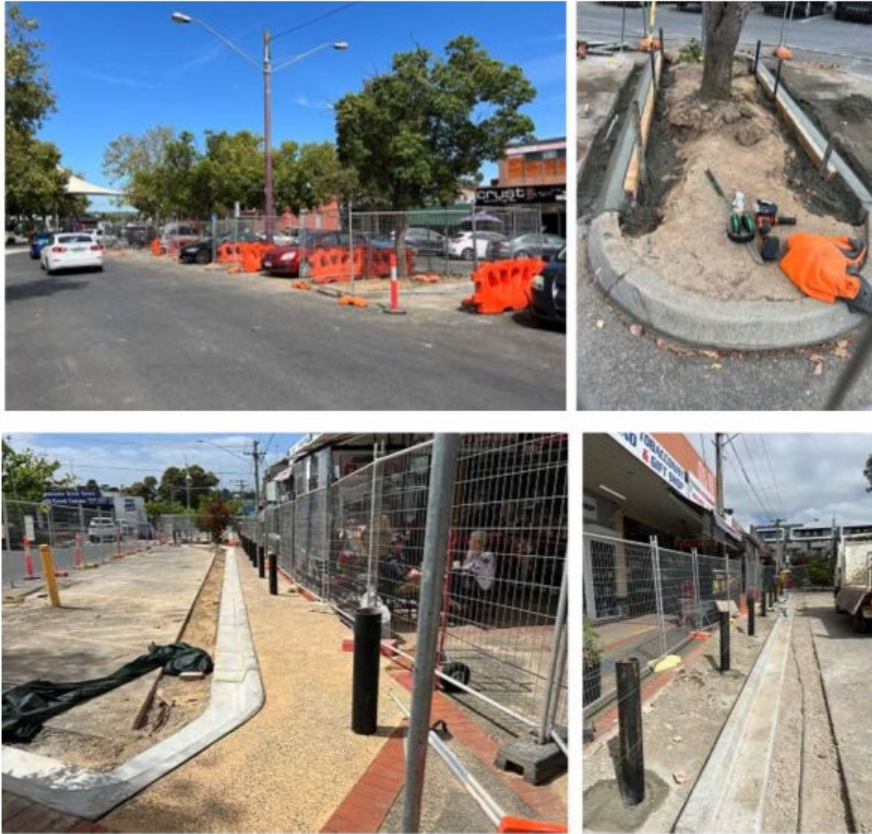
The Streetscape Program including safety and amenity works at; Macedon Square, Tunstall Square and Jackson Court is on track and/or approaching completion.
